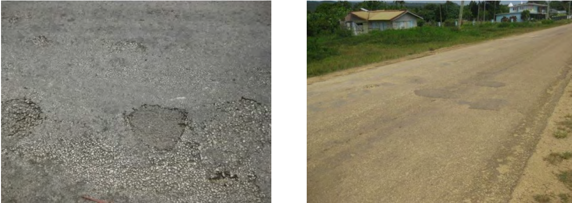
Figure 5 Pothole Patches on Hihifo Road and Pothole patches on 'Eua District
