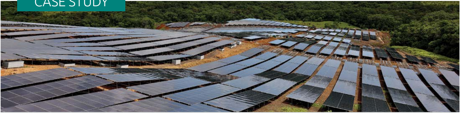
Palau solar plant. Credit: DFAT
