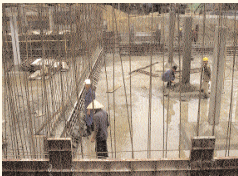
Construction work underway for new water treatment plants in Vietnam. Photo: Tim Acker
