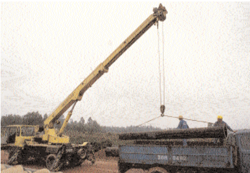
Construction work on track to bring clean water to five Vietnamese towns by the year 2000. Photos: Tim Acker
