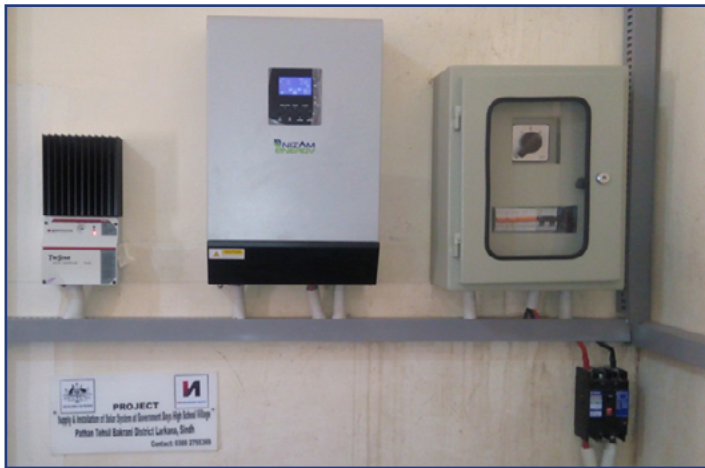
Source: Australian High Commission, Islamabad Meeting ends through alternative means—the Direct Aid Program funded the installation of solar energy generation infrastructure at a public school, Larkana (Sindh, Pakistan).
