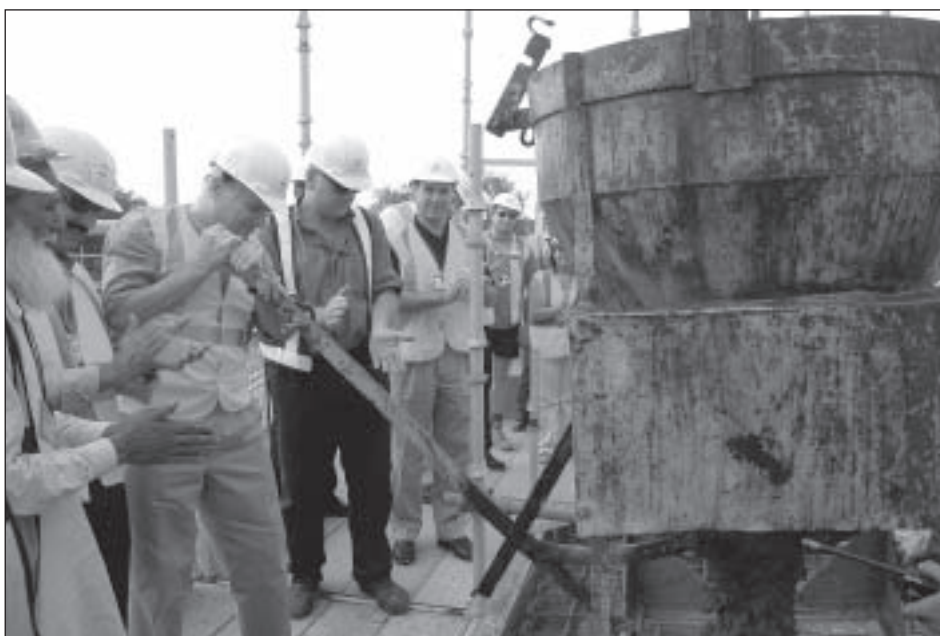
High Commissioner to India John McCarthy (third from left) initiates the final concrete pour to top out works on the new chancery building in New Delhi.
