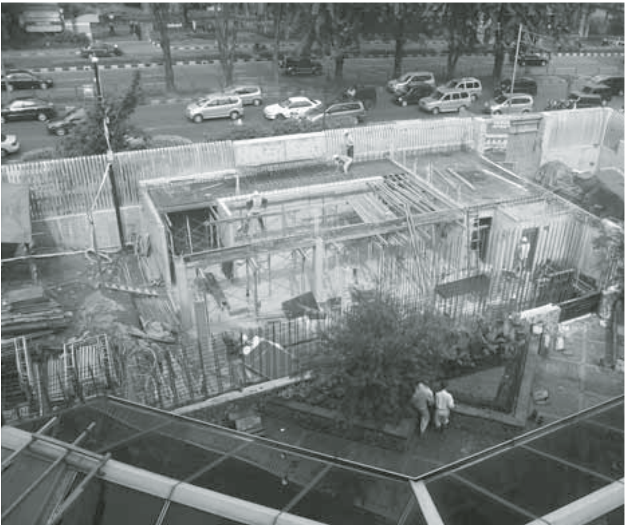
Repairs to the Australian embassy Jakarta and additional security works under construction following the terrorist bombing in September 2004.
