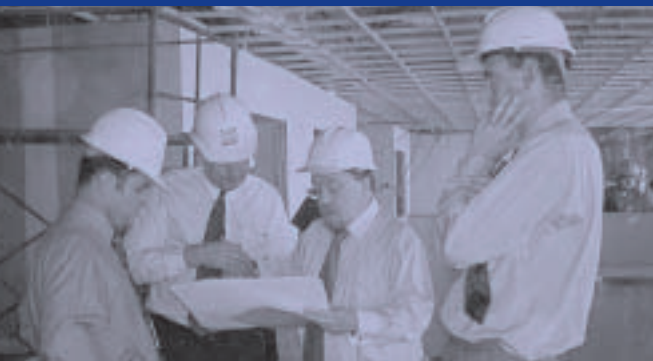
Embassy staff inspect the layout of the new chancery in Manila, which was completed in May 2003. From left to right: Alan Morrell, Austrade Senior Trade Commissioner in the Philippines, Mike Moignard, Austrade Executive General Manager South East Asia, departmental staff member Jamie Troup, and Miles Armitage, Deputy Head of Mission, Manila.
